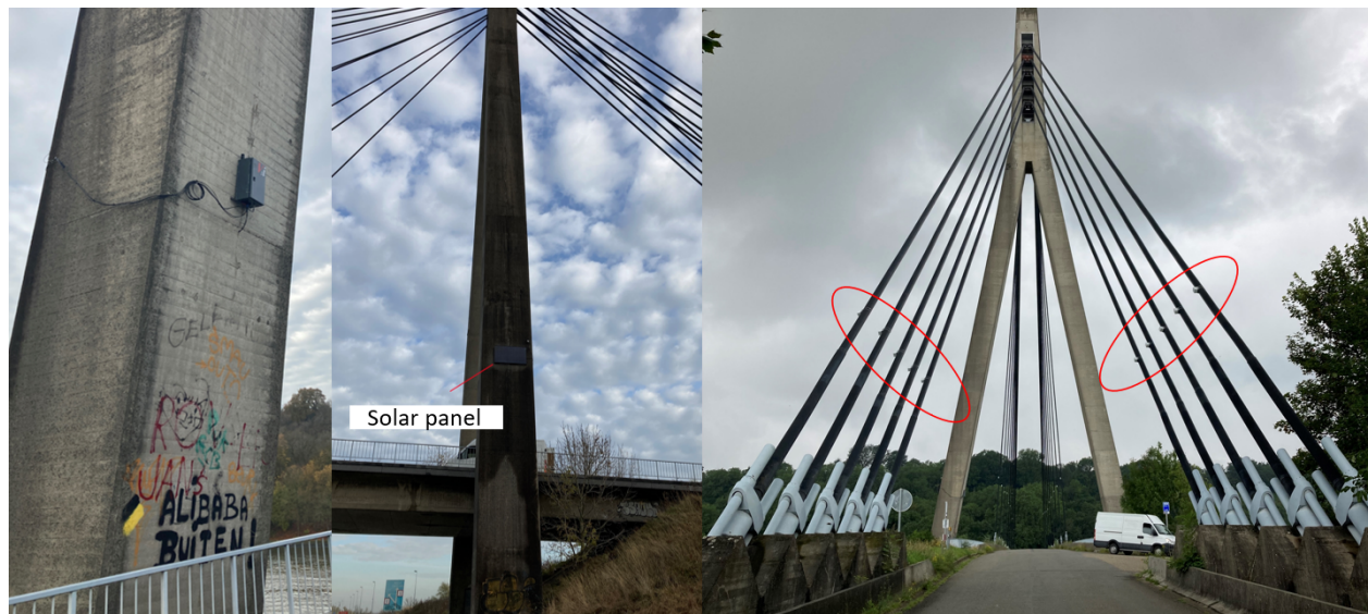
Figure 7: Photographs of the LYRA system attached to the Lanaye bridge showing the central station (right), the solar panel (center) and the wireless nodes attached to cables LG11 to LG15 and MA11 to MA15 (right)
