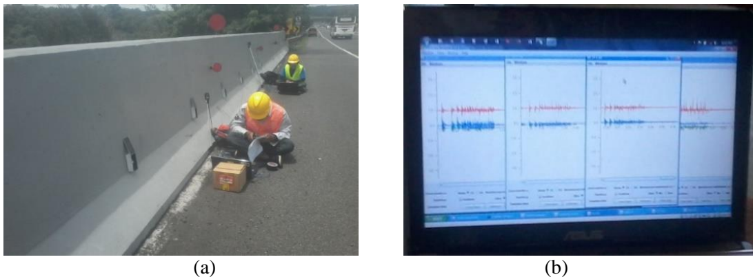
Figure 3: (a) Installation of the accelerometer sensor on the side of the bridge (b). Sensor-detected vibration response display
